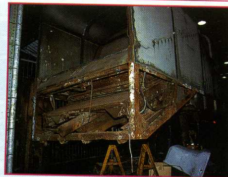
The underside of the loading hopper, revealing the extent of the corrosion to the basic steel structure under the aluminium panels.
