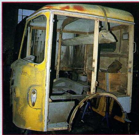
The cab on its return from the sandblasters and awaiting repairs to the timber work. There's still a long way to go yet!
